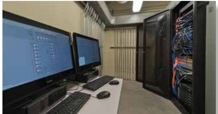
The new 433,409-square-foot Orleans Parish Sheriff's Office in New Orleans opened in 2015, with the SEC work completed by CCC Group.
